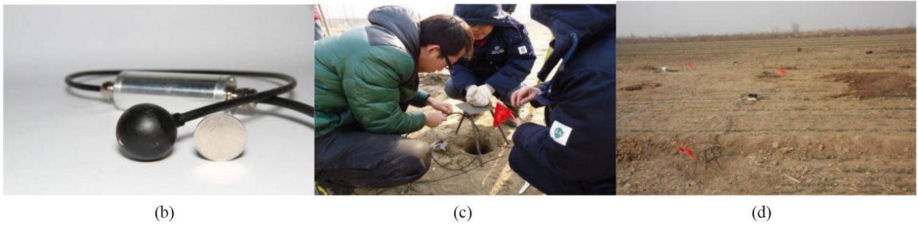
Notes: (a) Schematic of sensor layout; (b) an omnidirectional vibration sensor; (c) installing sensors; (d) sensors laid out
