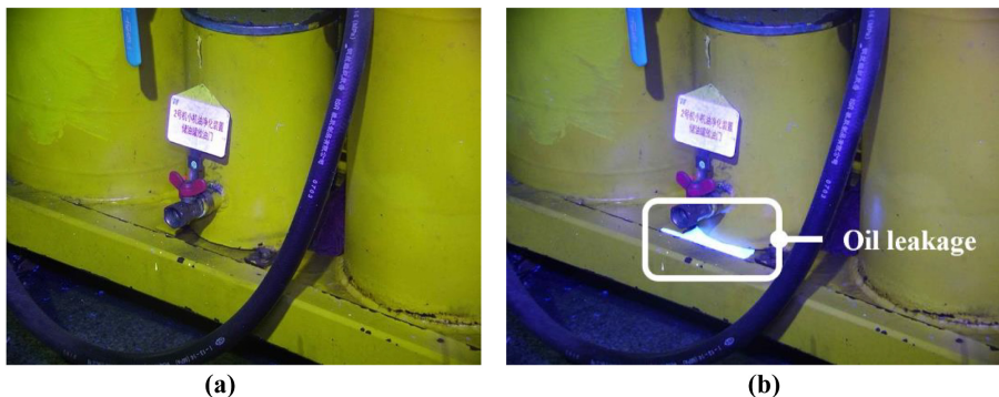
Figure 2. Oil leakage under various sources of light: (a) visible light; (b) UV light
