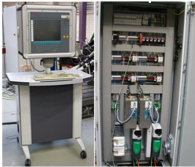
Figure 11 Control system hardware
